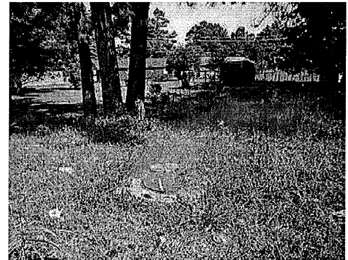
Defective Manhole Eastside Basin, Manhole D6
